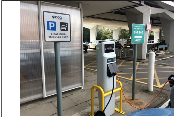
Figure 1 EVCP at Barnet House
